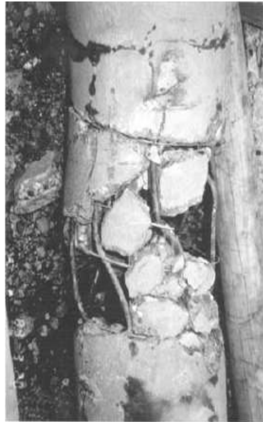
Fig: 13 A Pile Damaged by lateral Ground Displacement During 1964 Niigata Earthquake (Yasuda et al, 1999)
